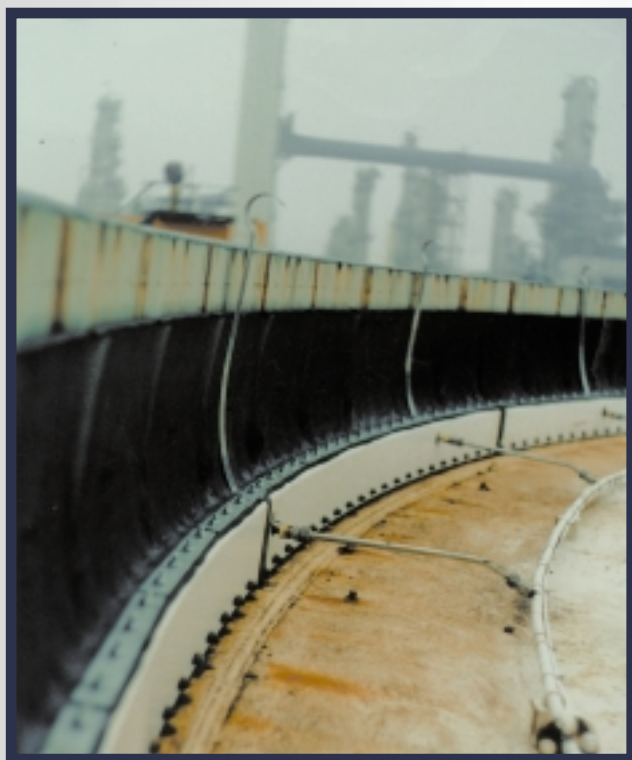
CTS10 seal on rim extension with fire detection system.
