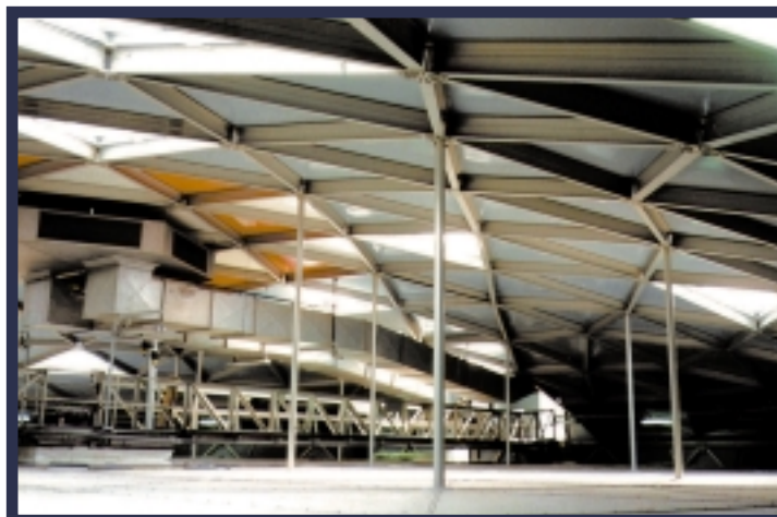
Suspended low cover from dome structure, to reduce vapour volume to be treated.
