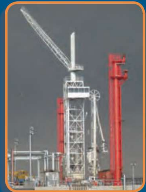
Multipurpose gangway tower with liftplatforms, telescopic gangway, hydraulic stores crane, control cabins and fire monitor columns. Shanghai - China
